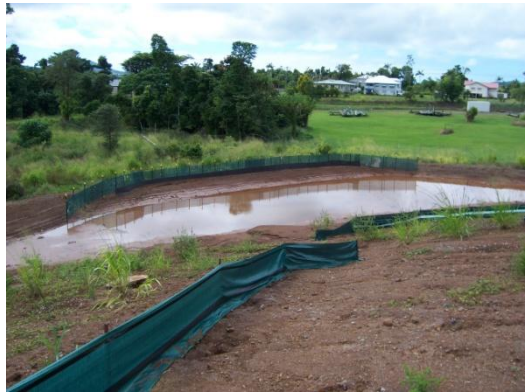
Erosion and Sediment Control – Goondi Bend
